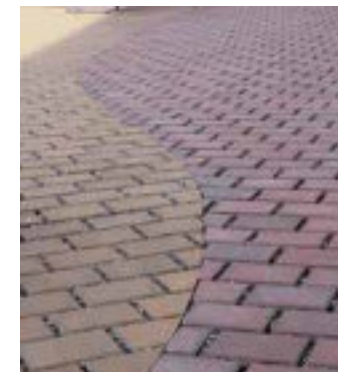
Figure 90: Permeable brick paving.
