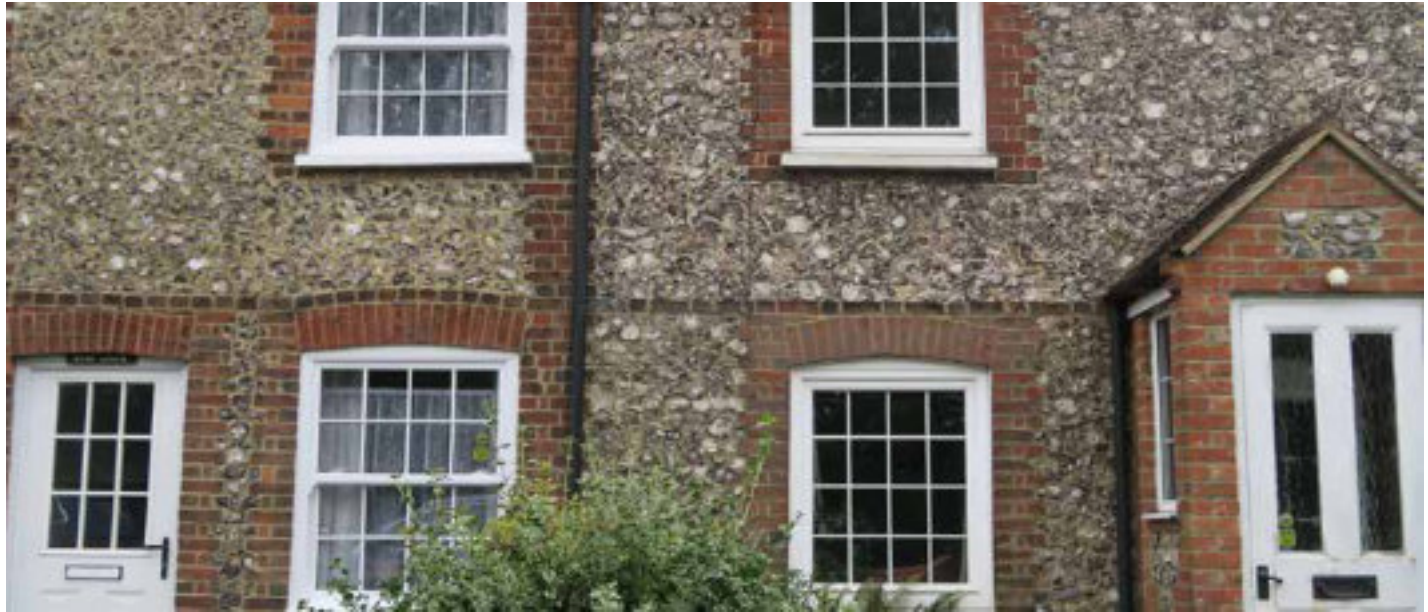
Figure 69: Façades with consistent arrangement of multi-pane windows with attractive brick ornamentation and articulations.
